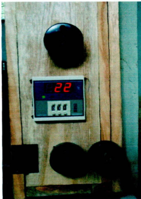
Fig. 3.11: Switch board of the dryer
