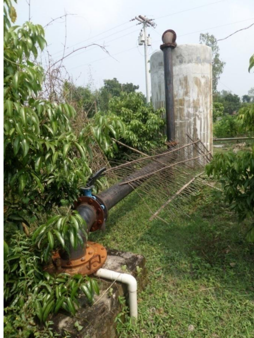
Fig. 3.3: Tank used for Burried pipe irrigation line
