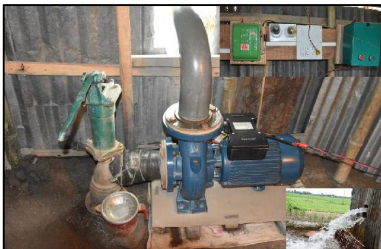
Figure 3-9: Electric Pump at Panchagarh District
