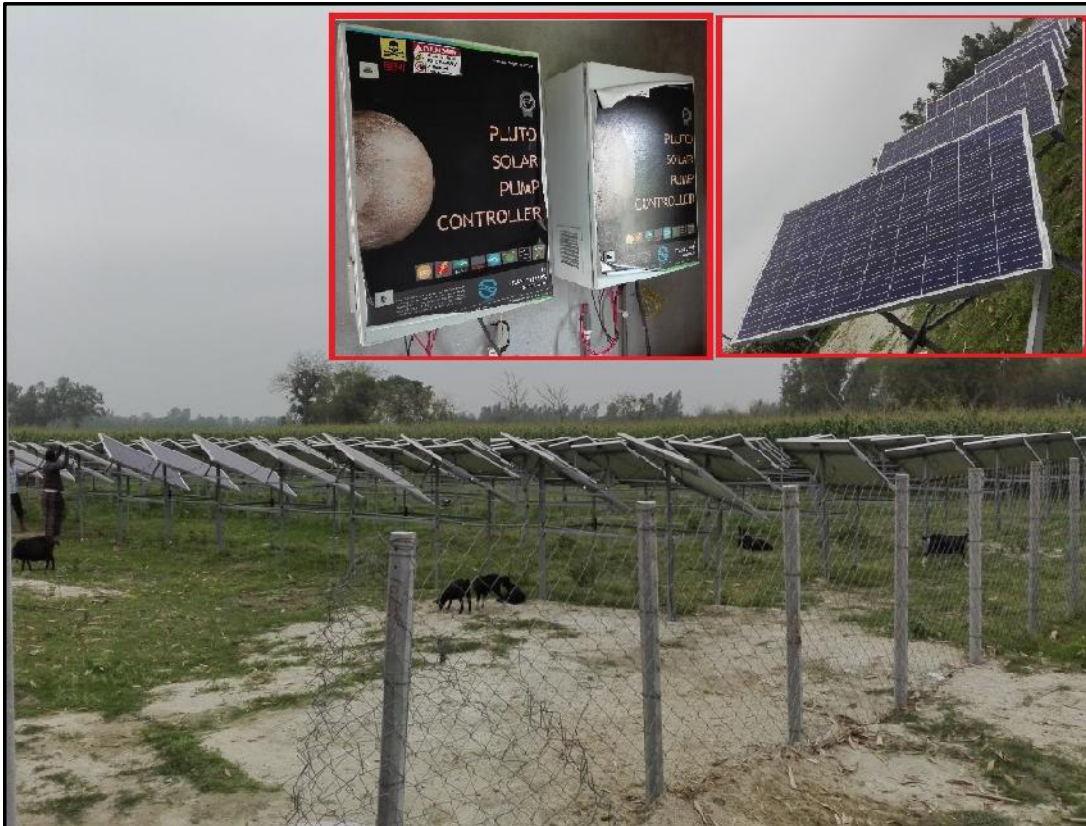
Figure 3-10: Solar Pump plant at Dinajpur District
