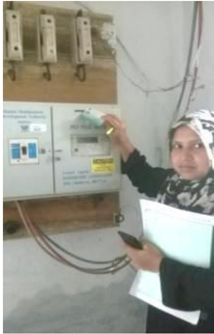
Figure 3.3: The procedure of inserting prepaid card in the slot of prepaid meter
