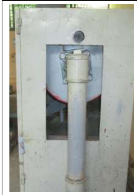
Fig-3.5: Hot air supply pipe
